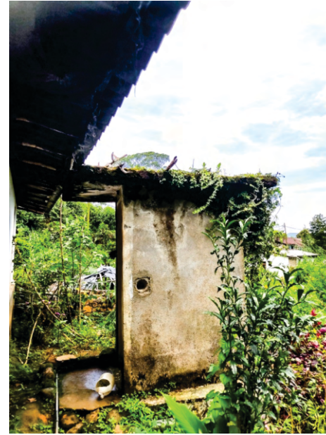
Inadequate sanitation facilities
